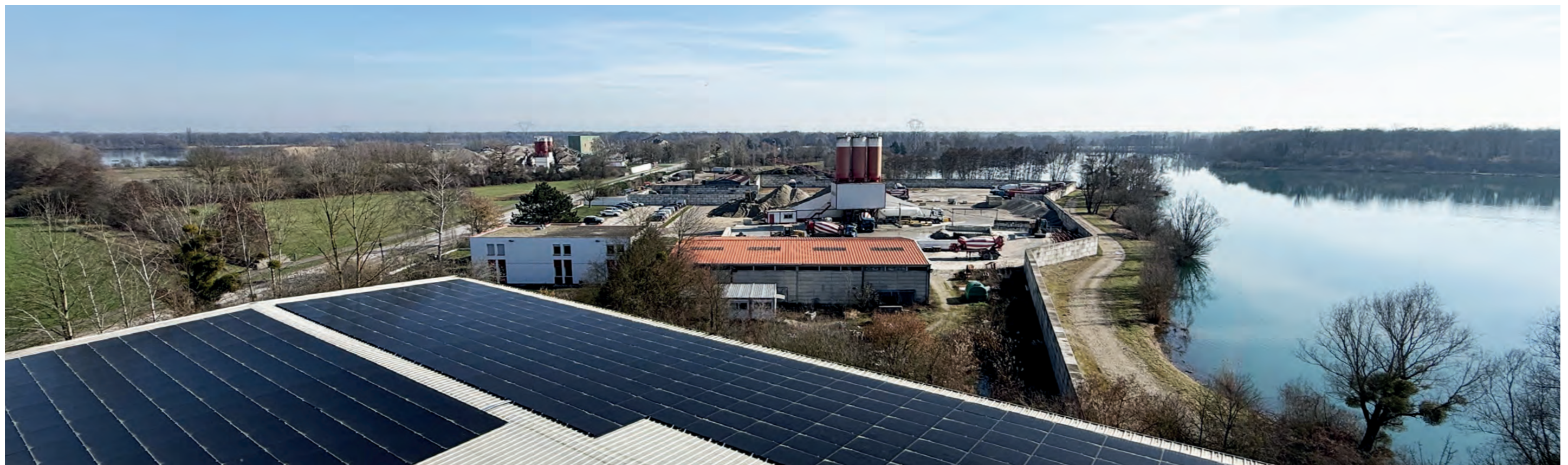
Photovoltaikmodule in Krautergersheim
